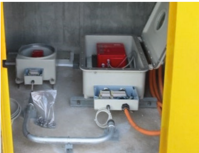
Seismic instrumentation on a liquid gas plant in explosion-proof design
