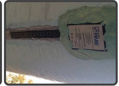
matPIMS™ 1x15 array permanently installed using viscoelastic putty to overcoat sensor strip and head before wrapping/backfill.
