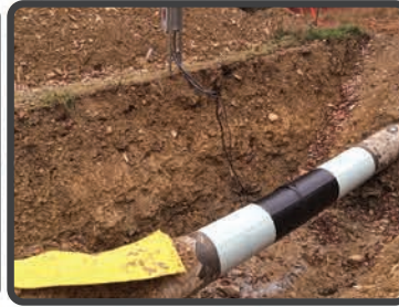
Fully coated and wrapped installation with RS-485 cable mounted in test station for data collection.
